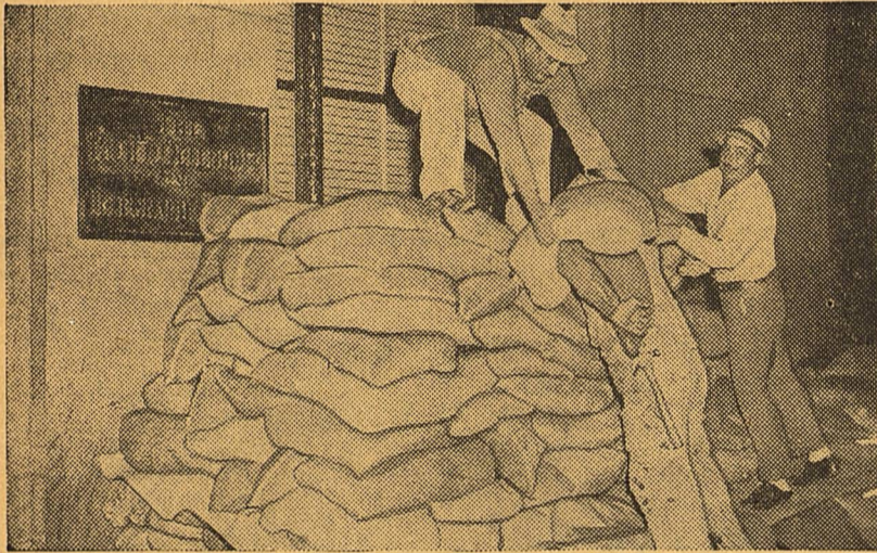
Following almost nightly air raid alarms and blackouts of San Francisco since the start of the war, the Pacific Telephone and Telegraph company has installed a sandbag barricade across the front of their building. Workmen are shown here erecting the wall of sandbags, which will protect vital telephone equipment from possible enemy bombs.
