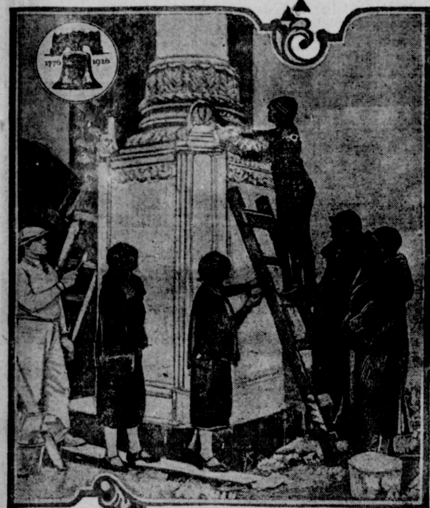
Young women artists turn from their jars of color and paint brushes to assist plasterers in setting ornaments in place atop huge pylons which adorn the main entrances to the Palace of Agriculture and Food Products, of the vast exhibition buildings which form a part of the great Sesqui-Centennial International Exposition being staged in Philadelphia from June 1 to December 1 to celebrate the 150th anniversary of the signing of the Declaration of Independence. Climbing ladders and walking along rickety scaffolds is nothing new to these young ladies, but each time they do it they get a thrill.
