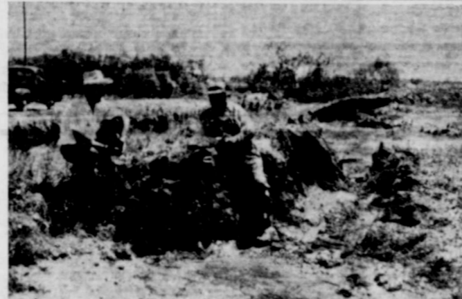
FLOOD DAMAGE —This photograph shows the damage done to a levee during recent hard rains in the Brown-Mills SCD. Runoff was too heavy during the rains and this levee gave away.
