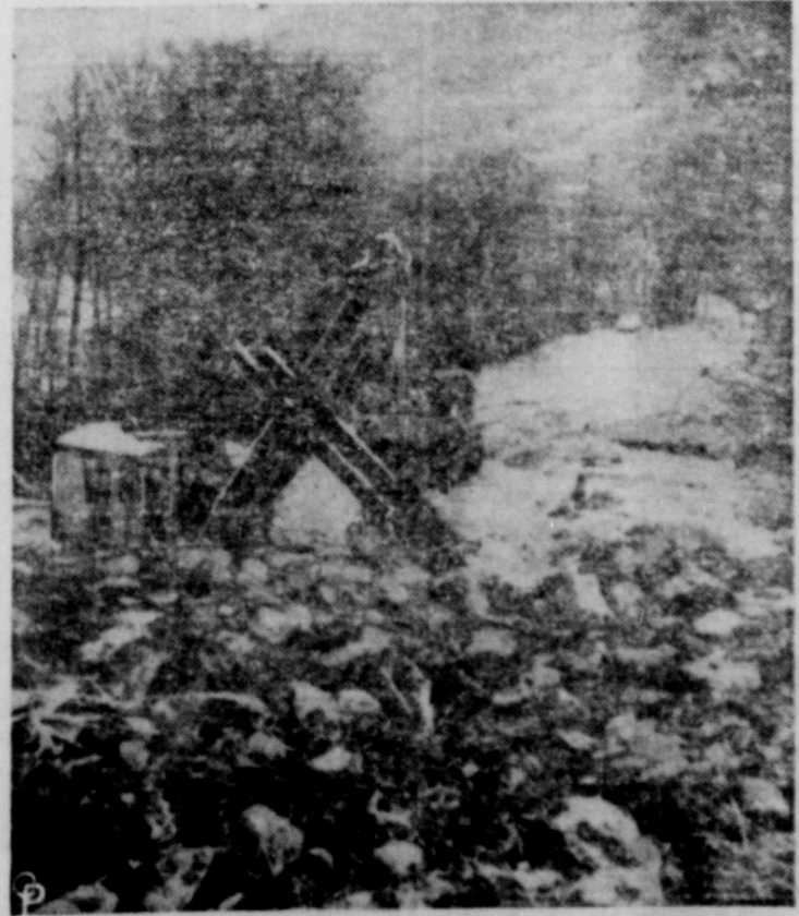
CLEAR ROCKSLIDE ROADBLOCK —A shovel goes to work on the avalanche of huge rocks that swept down a mountainside near Franconia Notch, N.H., blocking the main highway (background) between Boston and Canada with 28 feet of rubble. The rockslide, near the famous Old Man of the Mountains, followed torrential rains which touched off massive washouts in the White Mountain areas of New Hampshire.
