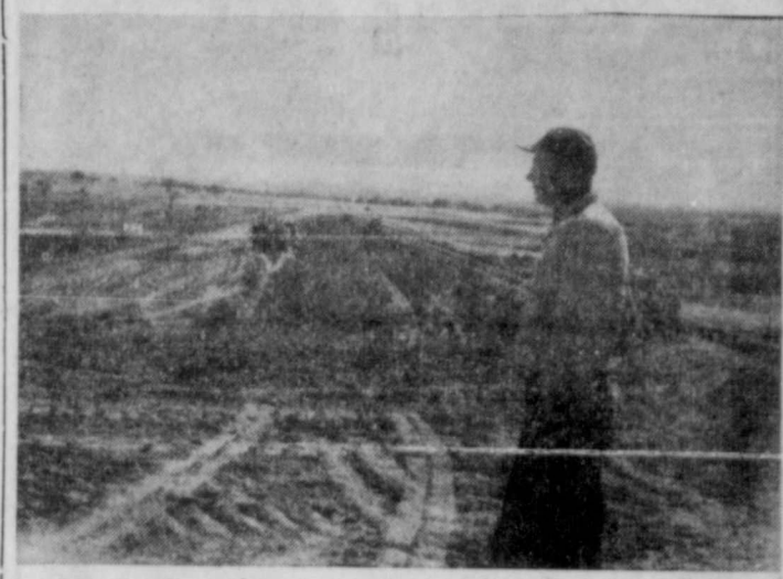
WATCHING DAM CONSTRUCTION —Dick Jones is shown here standing on top of the dam watching progress being made while construction moved ahead on the Site 17 A1 Blanket Creek flood prevention dam. —(SCS Photo)
