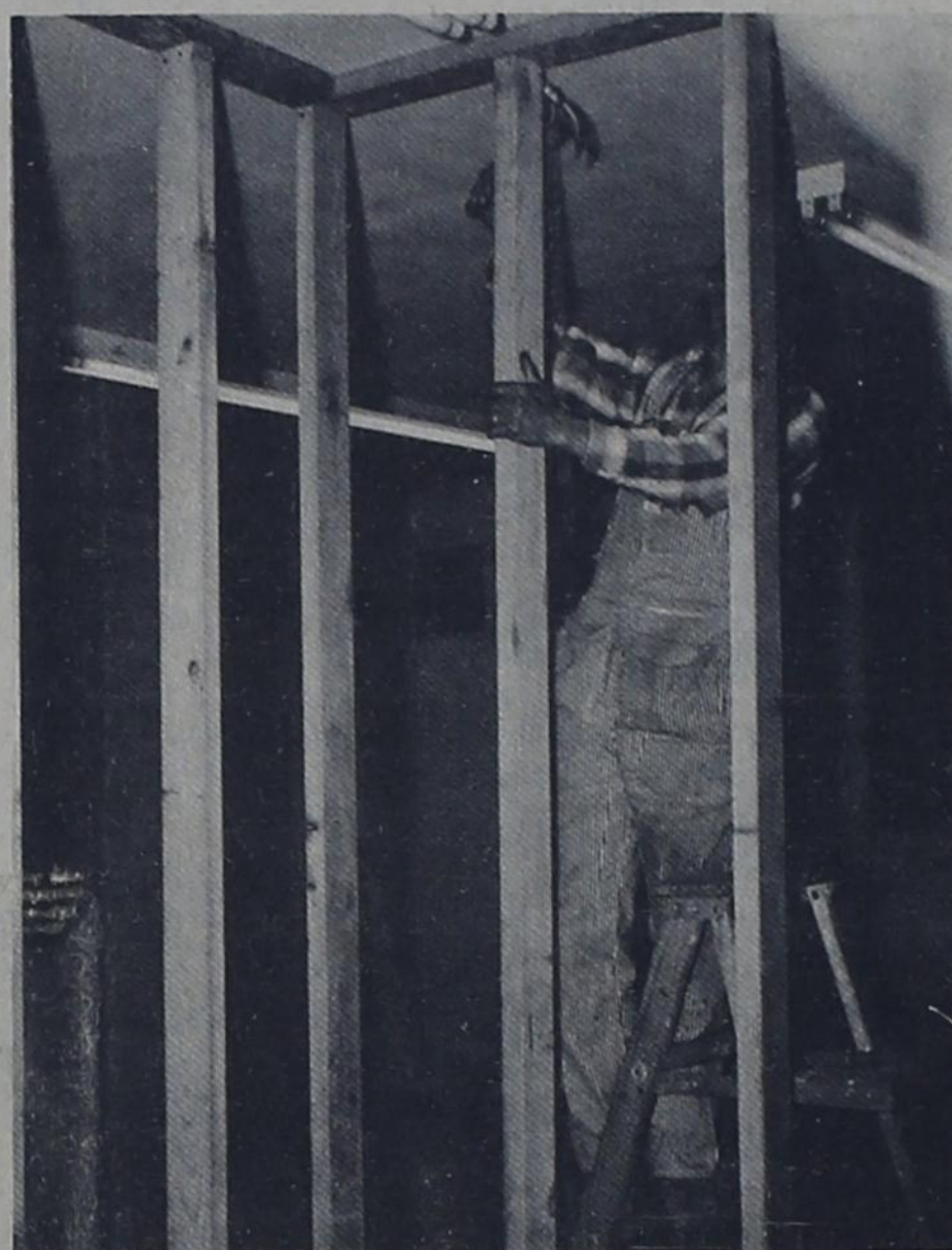
OFFICE BUILDING -- George Cervantez, Bovina carpenter, is constructing framework for the building owned by A. L. Glasscock on Highway 60 being remodeled for office space.
