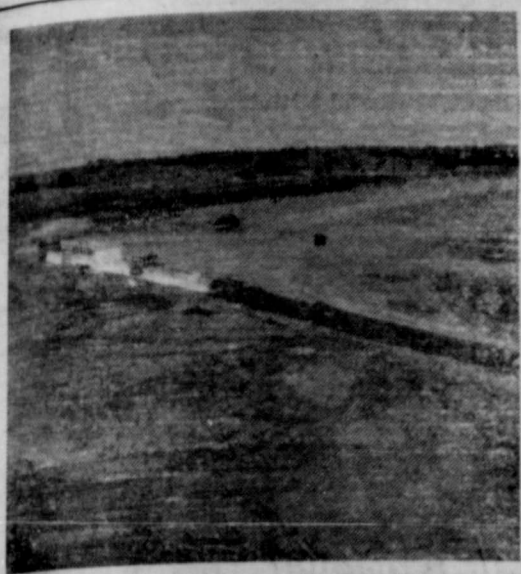
DRAWDOWN TUBE — Site six Northeast lateral being constructed on the Joe Beck Ranch two miles northeast of Ebony in western part of Mills County. The 30 inch principal spillway (drawdown tube) is shown being constructed. Structures, such as drawdown tubes, provide many benefits to control pollution in Mills County. Sediment is controlled along with protection of fences, farm improvements and highways. It also provides the opportunity for recreation. —(SCS Photo)
