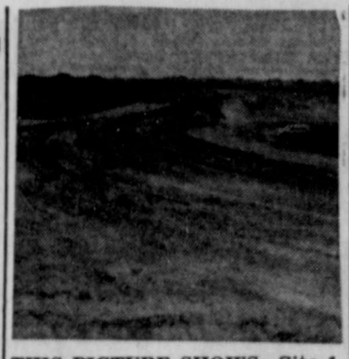
THIS PICTURE SHOWS: Site 1, Brown-Mullin Creek Watershed located some 3 miles North of Mullin on the M. E. Wylie Ranch. Site has been cleared, core trench has been dug and contractor, Fred Allen is back filling the core trench. —(SCS Photo)
