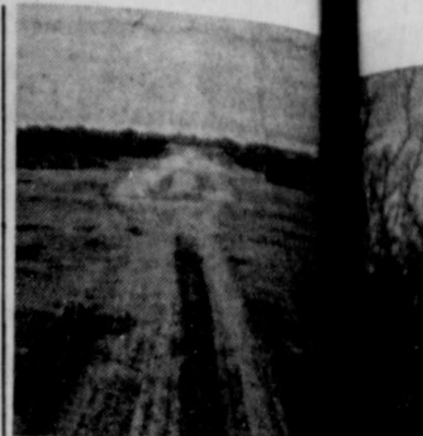
THIS PICTURE SHOWS: Site 2, Brown-Mullin Creek Watershed located on the Don Gee Farm four miles North of Goldthwaite. Site has been cleared and contractor, Lewis Lytle is starting to dig the core trench. —(SCS Photo)
