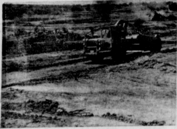
THE BROWN-MILLS Soil and Water Conservation District and Mills County Commissioners' Court are sponsors of the Brown-Mullin Creek Project. Contractor, Ford Allen, digging core trench on Site 2, Brown-Mullin Creek Project. This site is located on the A. G. Wasserman Ranch three miles Northeast of Mullin. —(SCS Photo)
