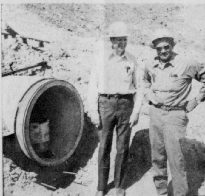
Charles Conrath and Eugene Williams observe the addition of another joint of concrete pipe as it is added to the draw down tube on Site 1, Bennett Creek.
