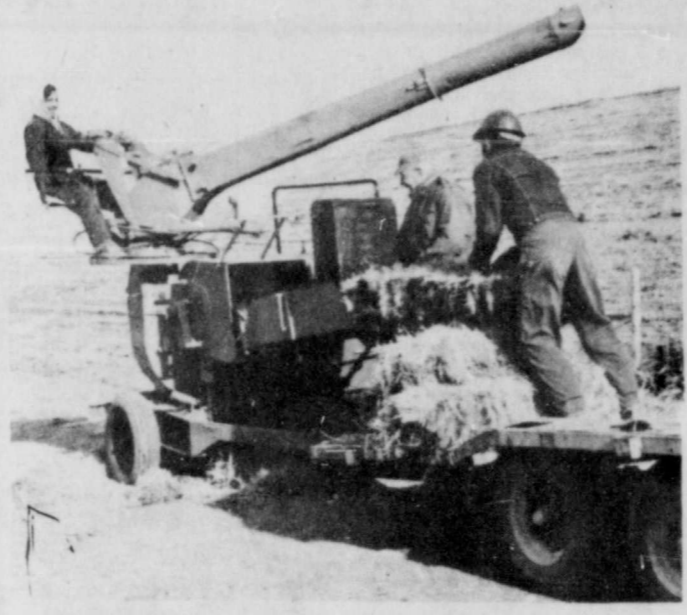
Erwin Brockmayer was the low bidder on vegetation of Sites 1, 2, 3, 4, 6 and 7 Brown-Mullin Creek Watershed Dams. Here Brockmayer blows hay mulch on Site 4 located on the Glover Dalton Farm six miles north of Goldthwaite. This mulcher cuts up the hay and blows it on the steep side slopes of the dam to hold down gully erosion and keep the seeded grass in place. — SCS Photo
