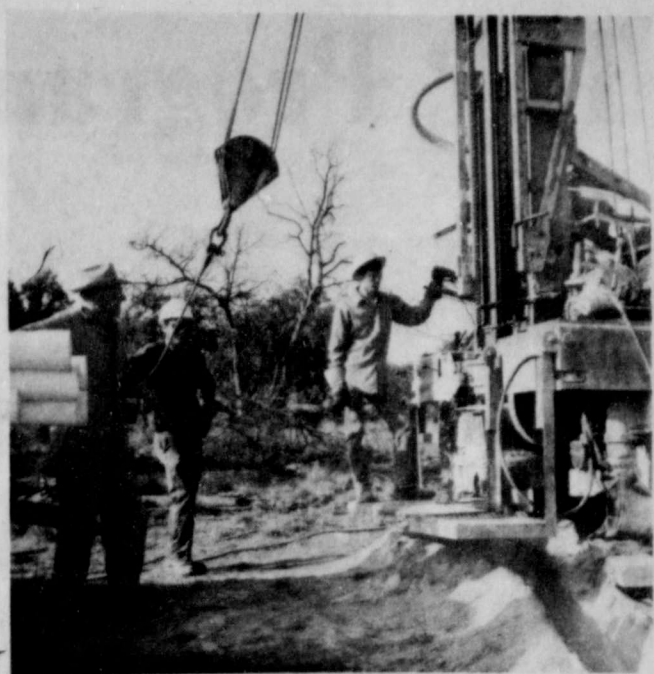
Erie D. Roberson well drilling operation on his place west of Goldthwaite. Water development is essential to realizing a conservation program. The Roberson well, to be used for livestock water by storage and by several pastures. Management systems can be utilized with the aid of proper water locations. — SCS Photo
