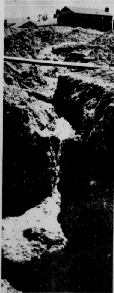
Some prior planning and application of simple conservation measures by the contractor and the lot owner could probably have prevented this severe erosion in a newly developed suburban area.
