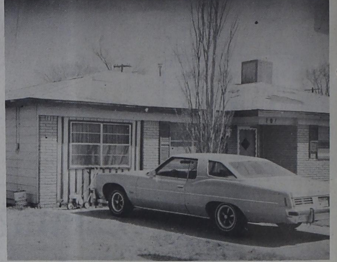
Pictured is the home of Richard and Evelyn Morris at 101 Boyce after the high winds Sunday took shingles off the front and side of their roof. Several reported damages to personal property. The picture window of the old Super Saveway building on Main Street was also destroyed. No injuries were reported. Winds blew at 40 and 50 miles per hour most of Sunday and Sunday night and continuing Monday.
