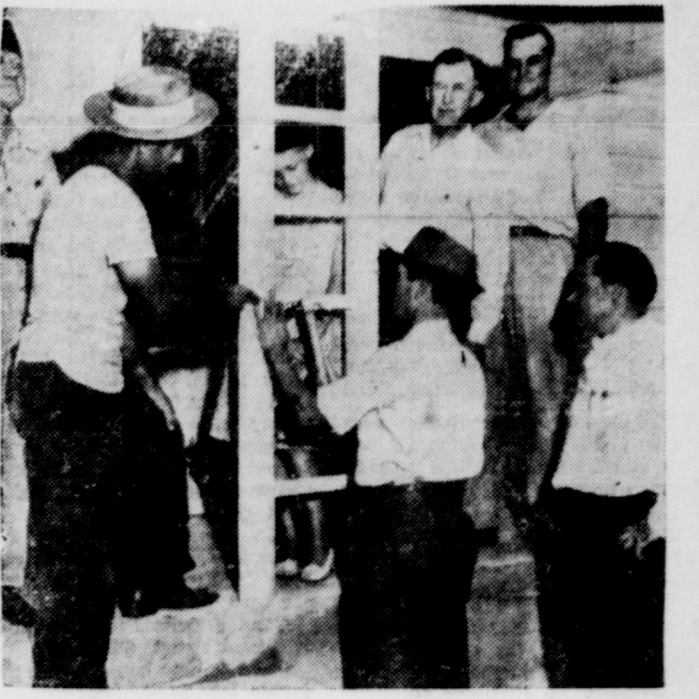
George Marquette, contractor, left, helps Jim Sanders, Houston blind vet, right, drive the last nail into his gift house which had been completed in the record time of three days in Houston, Texas. Watching Sanders, from left to right, are H. A. Hood, Adj. DAV; Sanders' daughter, Willie Mae; and construction officials J. L. Bryant, O. W. Rogers, and A. E. Gadberrry. (NEA Telephoto).
