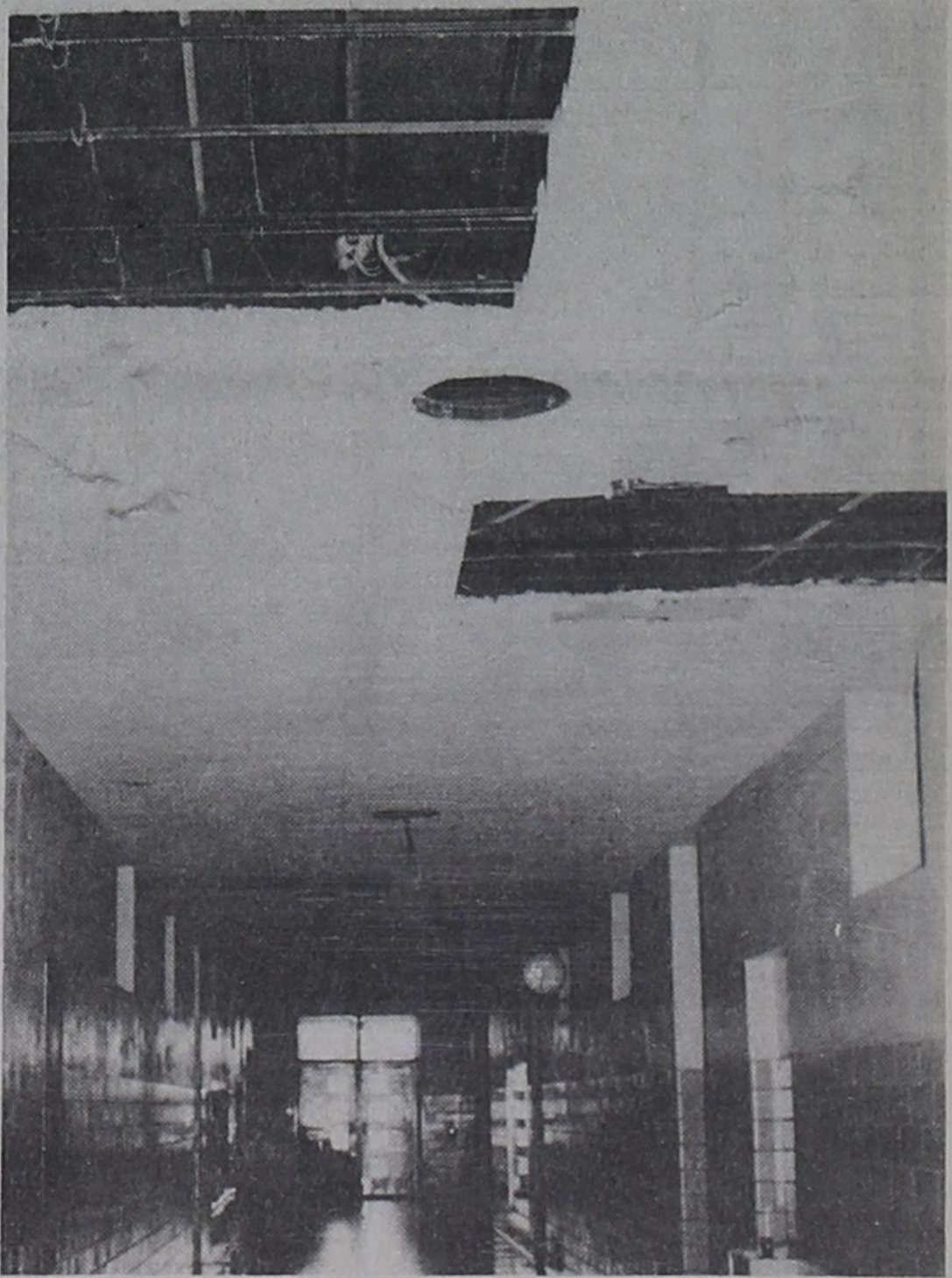
NEW CONSTRUCTION...Workmen are busy at Bovina School as central heating refrigerated air conditioning is being installed. The work will be completed when school starts the first week of September.
