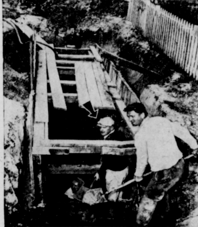
Keeping his campaign promise to provide a better sewer system, Raymond O'Brien (arrow), president of Hazelcrest Village, a suburb of Chicago, works in a ditch with other village officials. Working evenings and weekends without pay, O'Brien and his colleagues expect to save the community two-thirds of the usual cost of the job.
