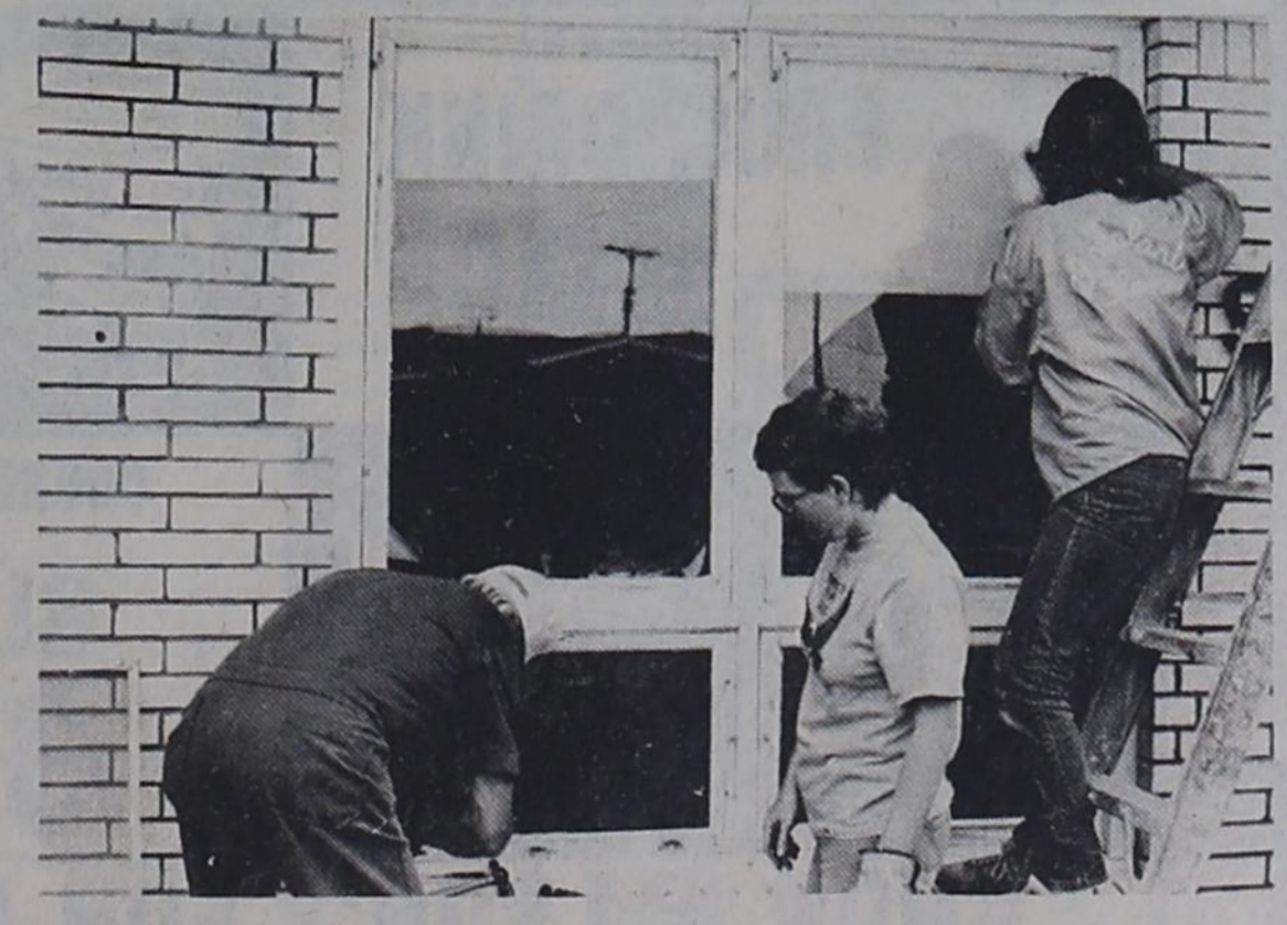
BROKEN WINDOWS....Friends and relatives help Carl Rea replace the broken windows at his home, located at 901 Avenue K. High winds
