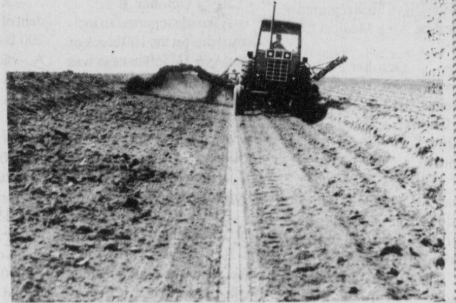
Constructing Terraces on sloping cropland helps control water erosion and conserves both soil and water.
