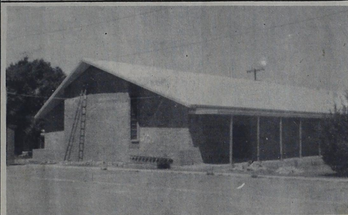
ALMOST COMPLETE -- Finishing touches are now being applied to new building of Bovina Church of Christ. The new brick structure is scheduled to be in use during first part of August. Shown here is south end of the L-shaped building.
