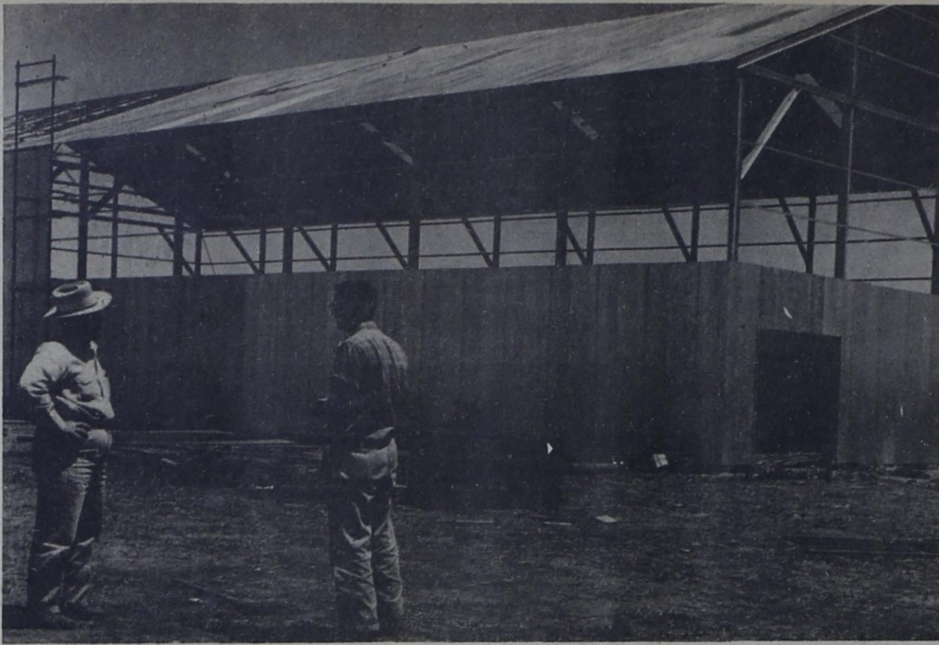
FRIONA'S NEW Farmers' Co-op Gin is rapidly taking shape two miles south of the city on state Highway 214. Completion of the gin is scheduled in time for this fall's crop. New manager of the gin, Jimmy Fletcher (right foreground) says he hopes to be able to gin a bale at the new gin by Sept. 15.
