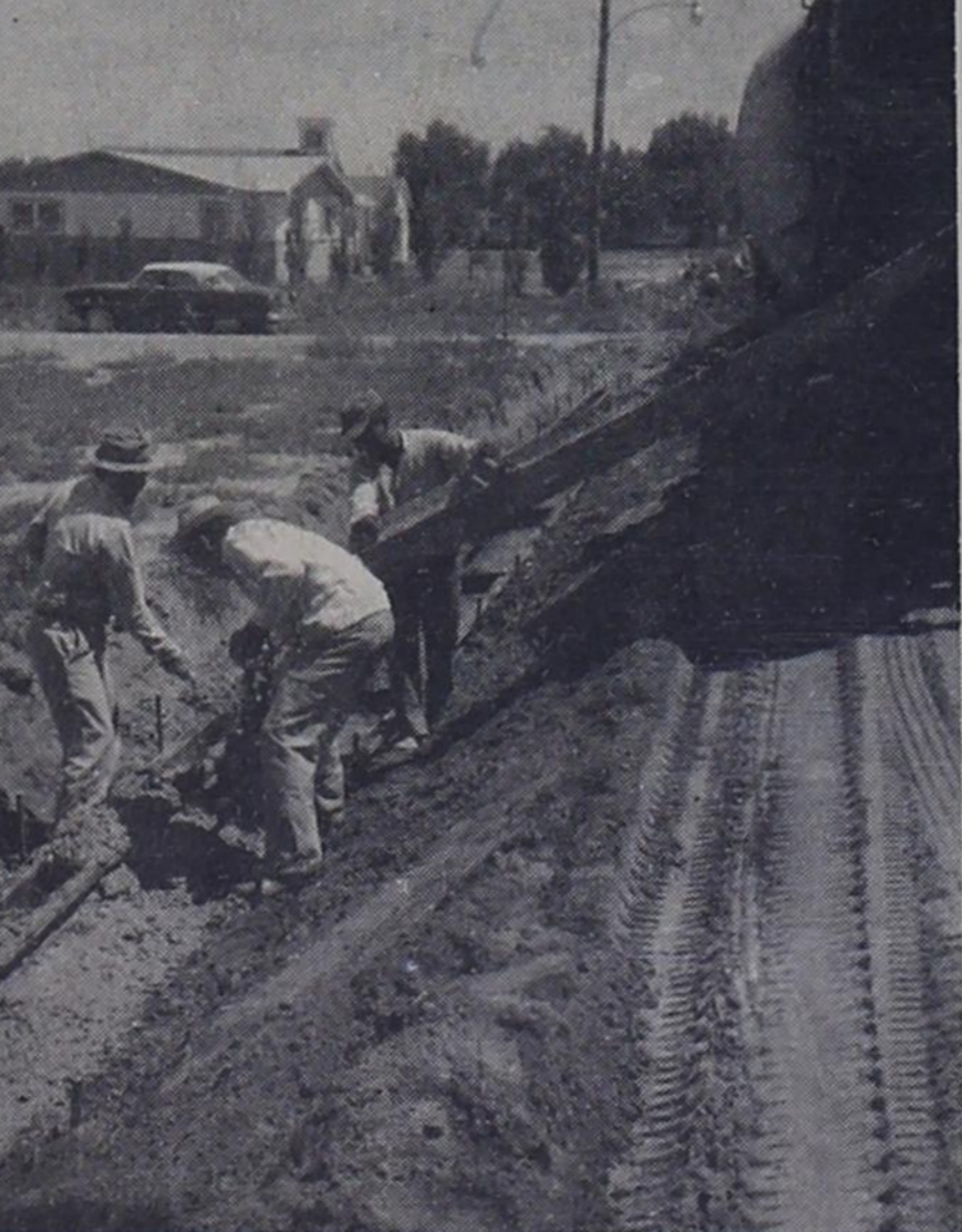
CURBS AND GUTTERS GOING IN -- These two scenes are now common in Bovina as Pioneer Pavers, Inc. of Lubbock are installing curbs and gutters on Third Street and Highway 86. Concrete is being poured into curb and gutter form at left. The three man crew at right is putting the finish on the still-wet concrete. Members of finishing crew are, left to right,
