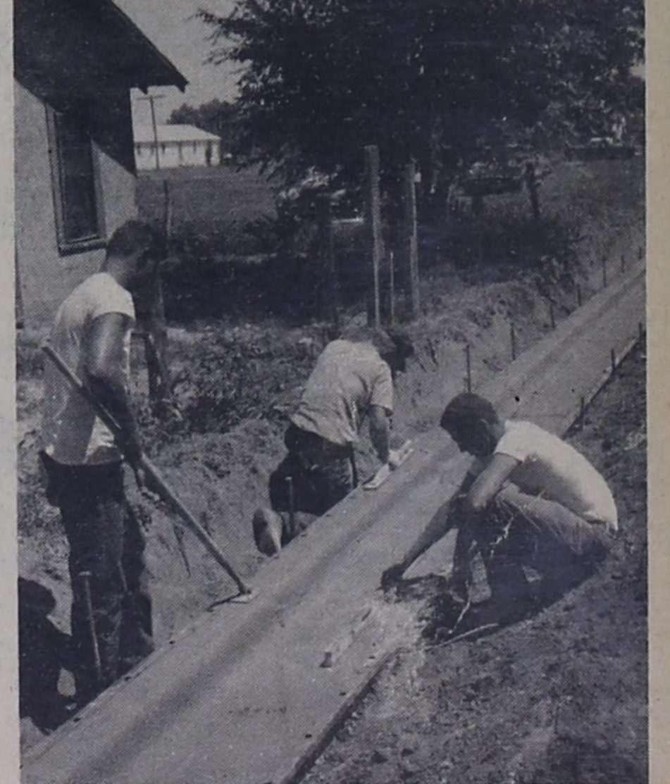
Patrick Hodges, Harold Satterfield, and James Cryder, all of Lubbock. Installation of some 20 blocks of curbs and gutters on state maintained streets and curbs, gutters and paving on some 20 blocks of residential streets is expected to take about six weeks.
