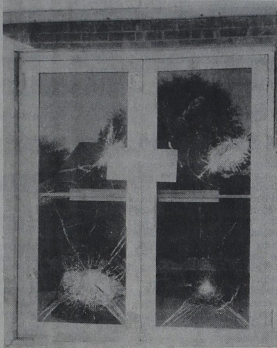
VANDALISM... Windows at the Bovina Post Office were broken out sometime early Sunday morning. Shown are the entry doors. The picture window on the front, and the side windows also were broken.
