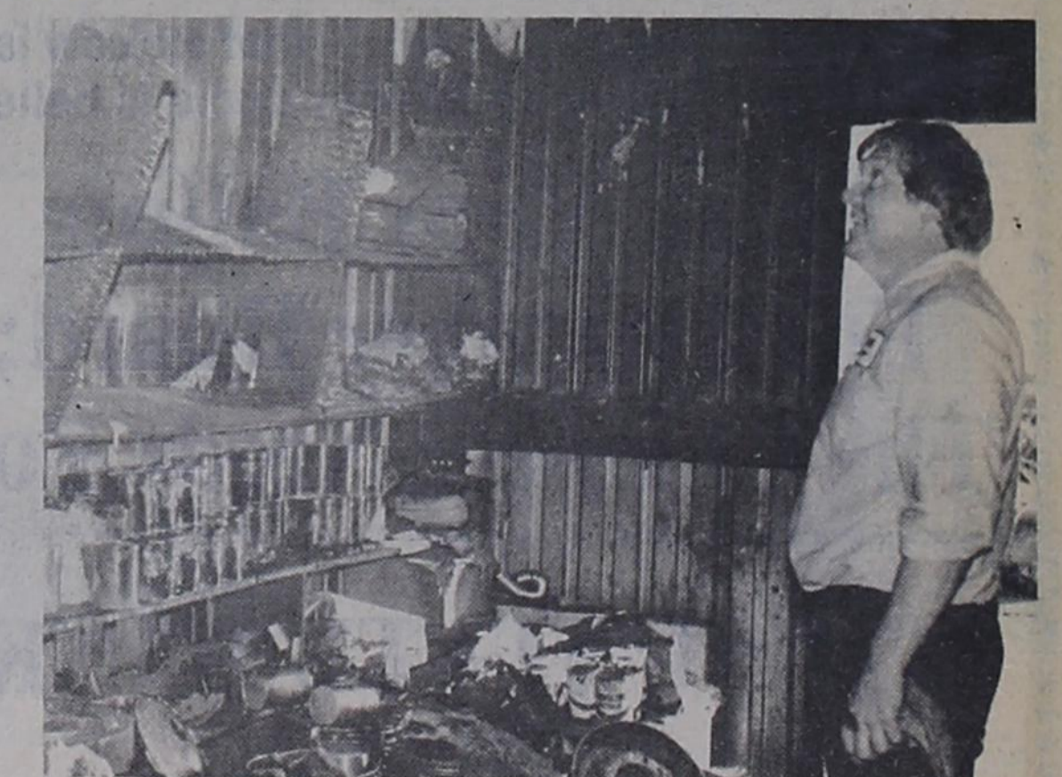
BLAZE DAMAGE... James Ritchie surveys the damage done when a fire swept through the Southside Motors last Friday.
