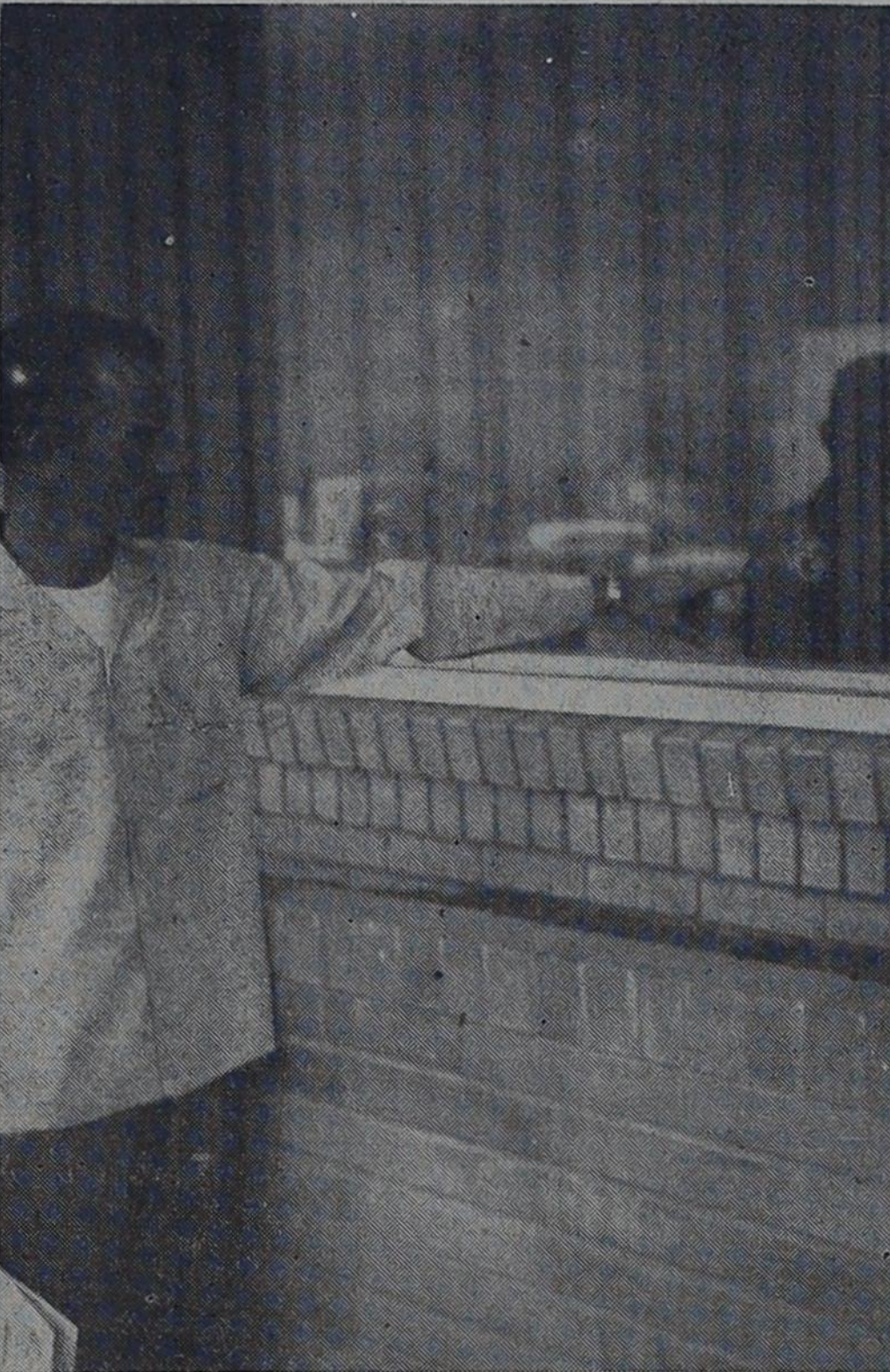
BULLET HOLES—Scott Levins obliges the cameraman by pointing to one of three bullet holes that were shot in the plate glass window of First National Bank Building Friday night. Another hole may be seen in the top center of the picture.
