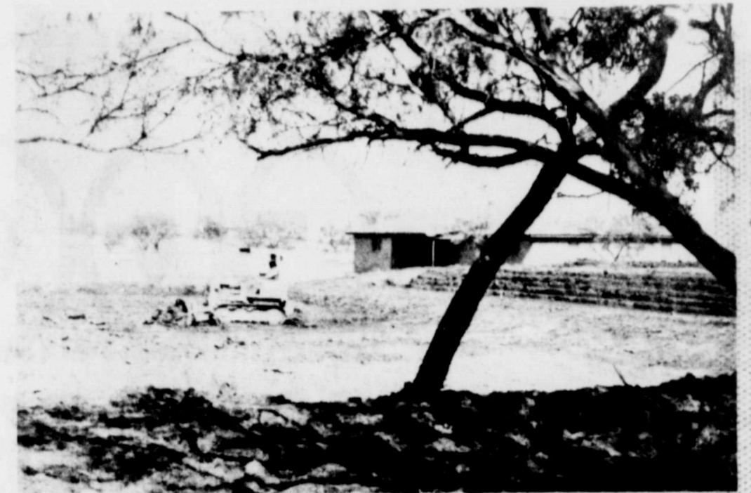
CONSTRUCTION--Work is under way on the new tennis court and leveling for the new townhouse to be built at the Merkel Country Club this week. The tennis courts will be 10 feet below the surface to allow for protection from the wind and to allow a clear view of the golf course.
