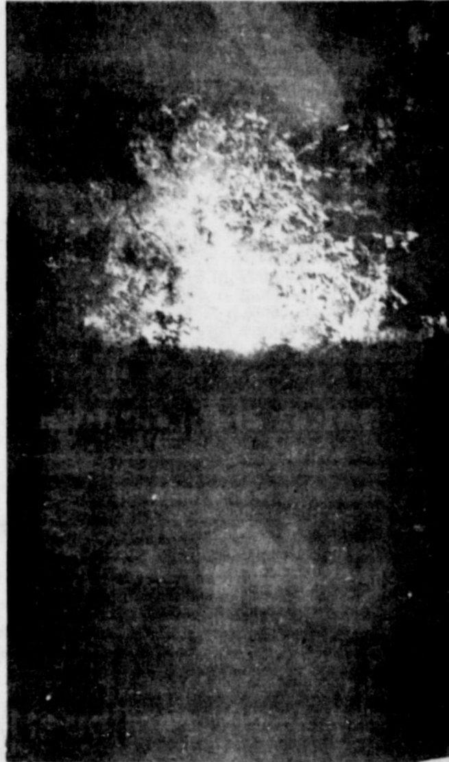
Sparks fly Thursday as two West Texas Utility lines cross. The crossed lines caused a two hour blackout over most of Merkel's east side, last Thursday. (Staff Photo by Cloy A. Richards)
