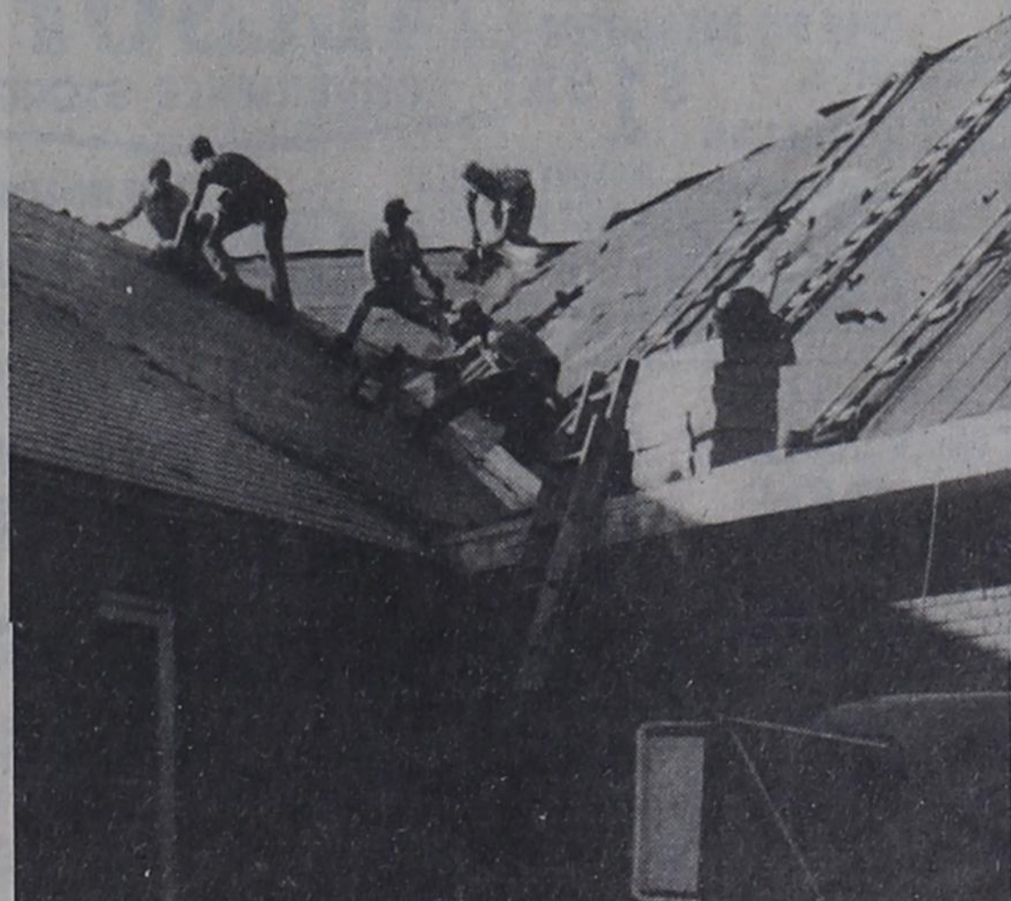
RE-ROOFING CHURCH.... rains and the workers have been busily working to finish the project before colder weather hits. Shown are workers who are re-roofing the First Baptist Church in Bovina. The process had been delayed by recent
