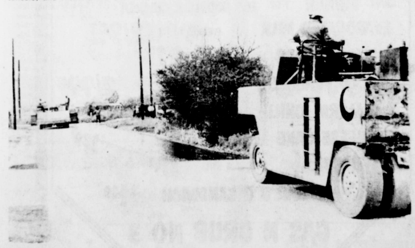
Nobles Construction of Colorado City found the weather fog for paving Saturday as they worked on the city's southside. The paving is being paid for by a fund secured by delinquent city taxes.
