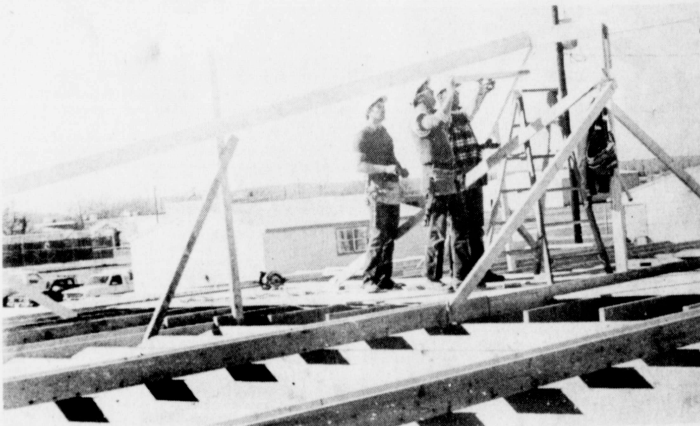
§ Work is moving along well on Merkel High. MISD maintenance construction work. the new Freshman Addition at crews are doing most of the [Staff photo]
