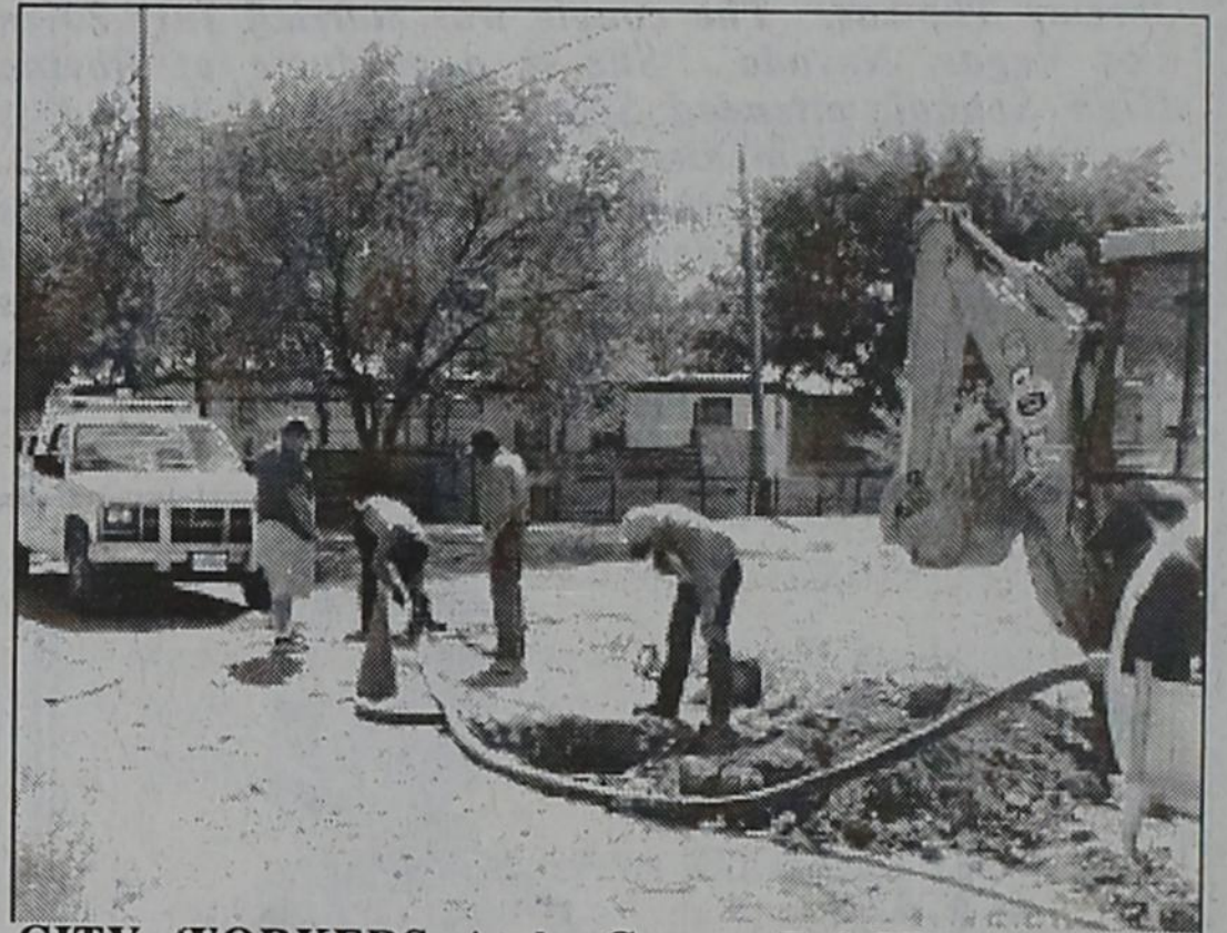
CITY WORKERS Andy Garza, Zef Villarreal and Caesar Marquez clear a major sewer blockage in the Gardner Addition on August 1. Monday, August 5, a water line break in the same addition left residents without water for about 7 1/2 hours. This city maintenance crew has been working hard to keep Bovina operating. photo by Ernest Terry
