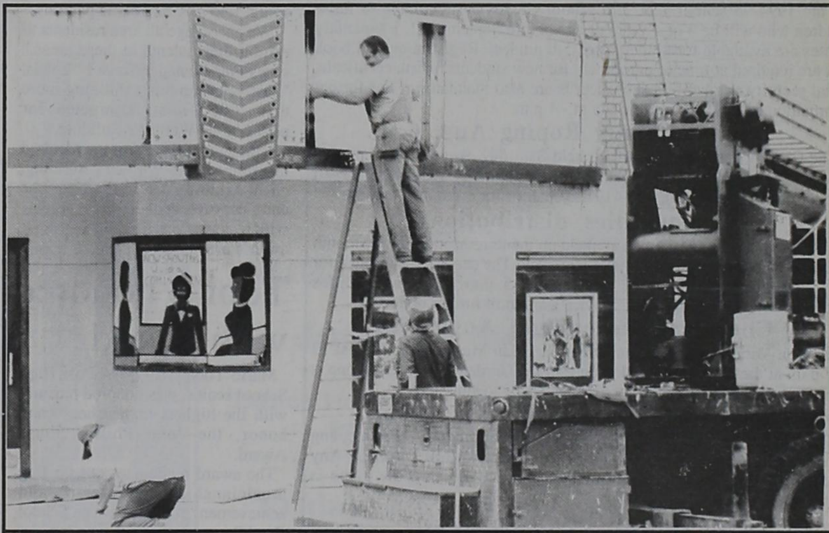
Hanging the last piece of plexiglass on the Tower theatre's marquee put an end to the renovation and a beginning to many shows that will appear in the newly remodeled theatre.
