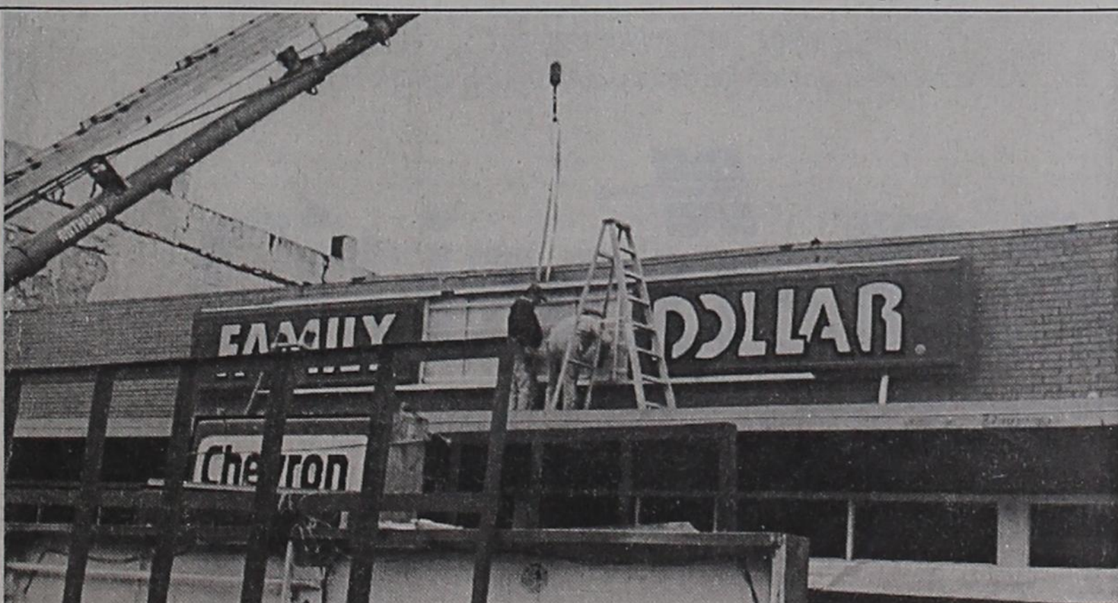
A new store sign was installed last week for Family Dollar Stores on East Main Street. Store representatives were here last week taking applications for an expected opening later this month. (Post Dispatch photo)
