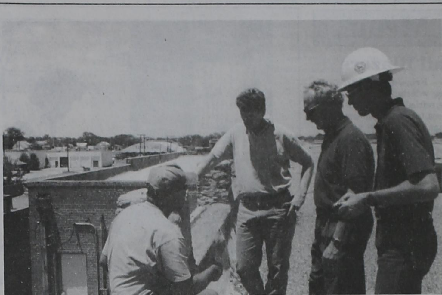
Inspecting the Algerita Building roof recently for a federal grant to make repairs to the historic facility were (left to right) Brock Jackson, Westex Roofing; Davis Melton, Tom Eisenhour and Ted Moore of Texas Department of Transportation.
