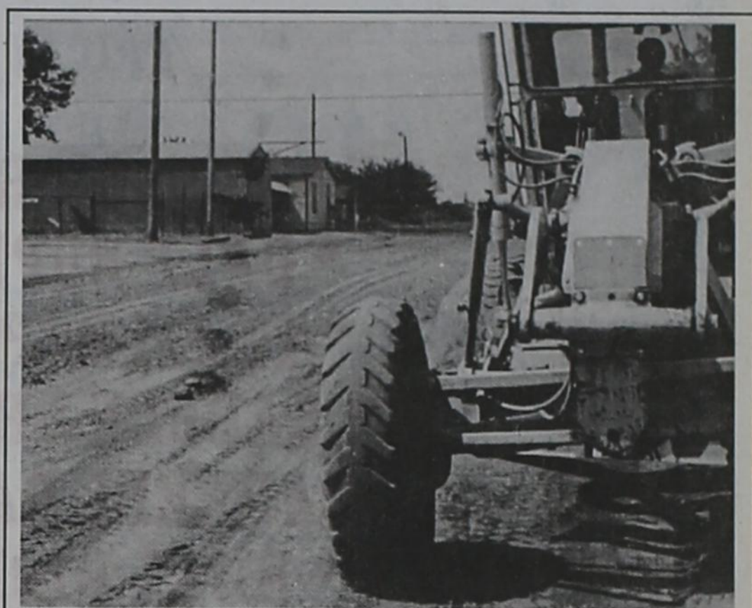
Post City maintenance crews are making improvements to approximately 15 city blocks of unpaved streets. Arnold Fry was grading and preparing a mix on the west side of town this week. City manager Fred Stephens said that crews will continue the work on a regular basis.
