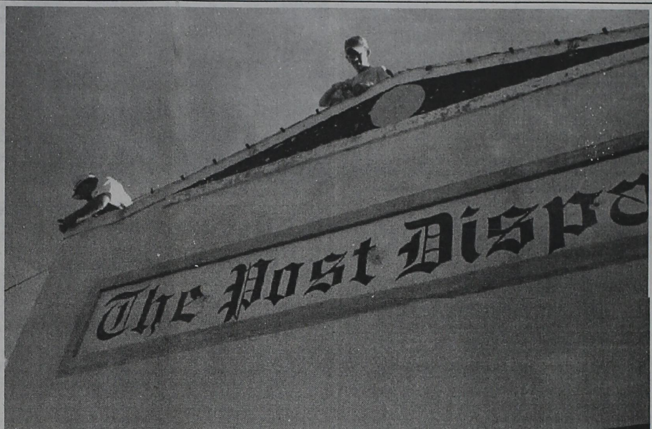
Rodney Tidwell (left) and Kyle Dunn, along with several other MAD DADS Inc. youth, were busy last week repairing broken lights on East Main Street buildings. The work is in preparation for this Saturday's Lighted
