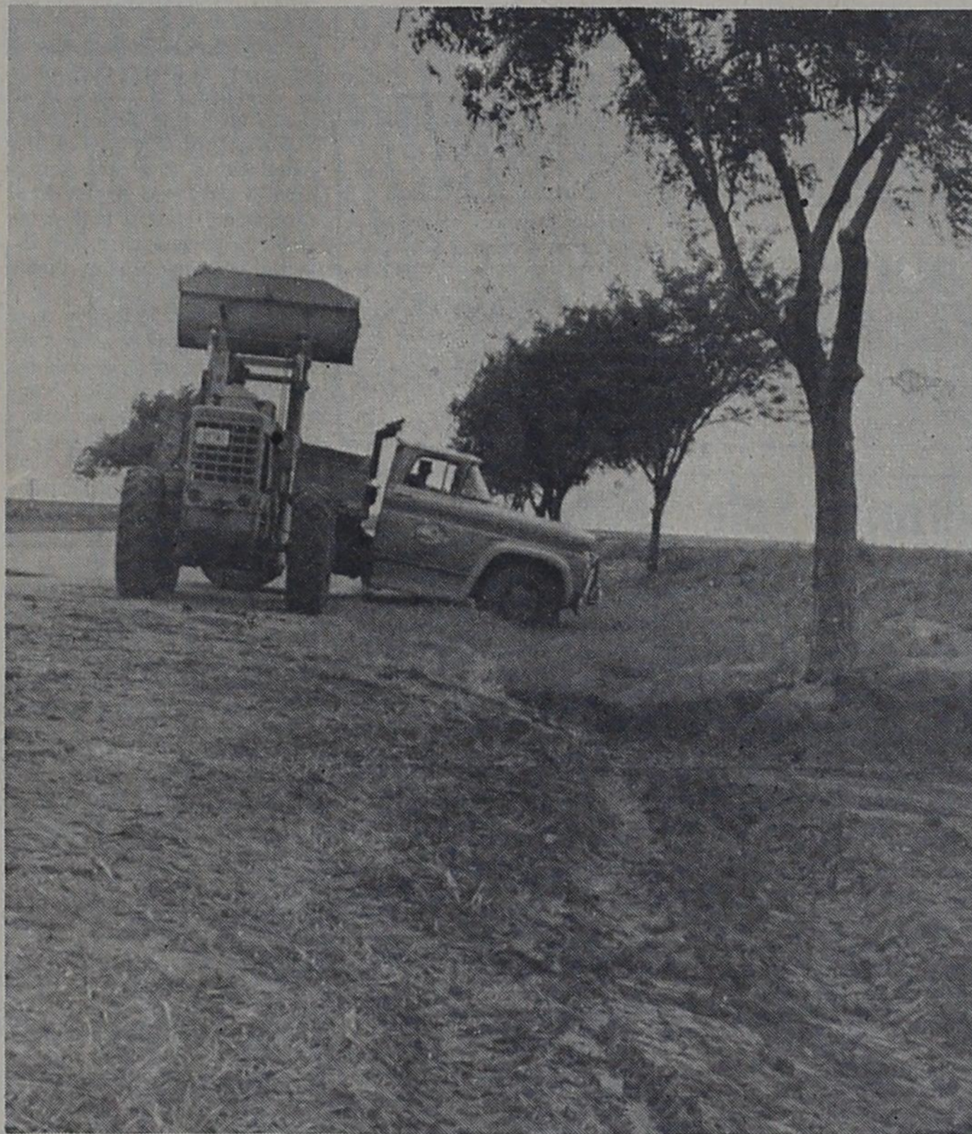
SCOOPING UP loads of what was formerly rich farm land, crews from the Highway Department dug out tons of rich soil from a highway borrow ditch last week. Some farmers were to use the soil for their lawns -- sort of expensive lawn dirt.
