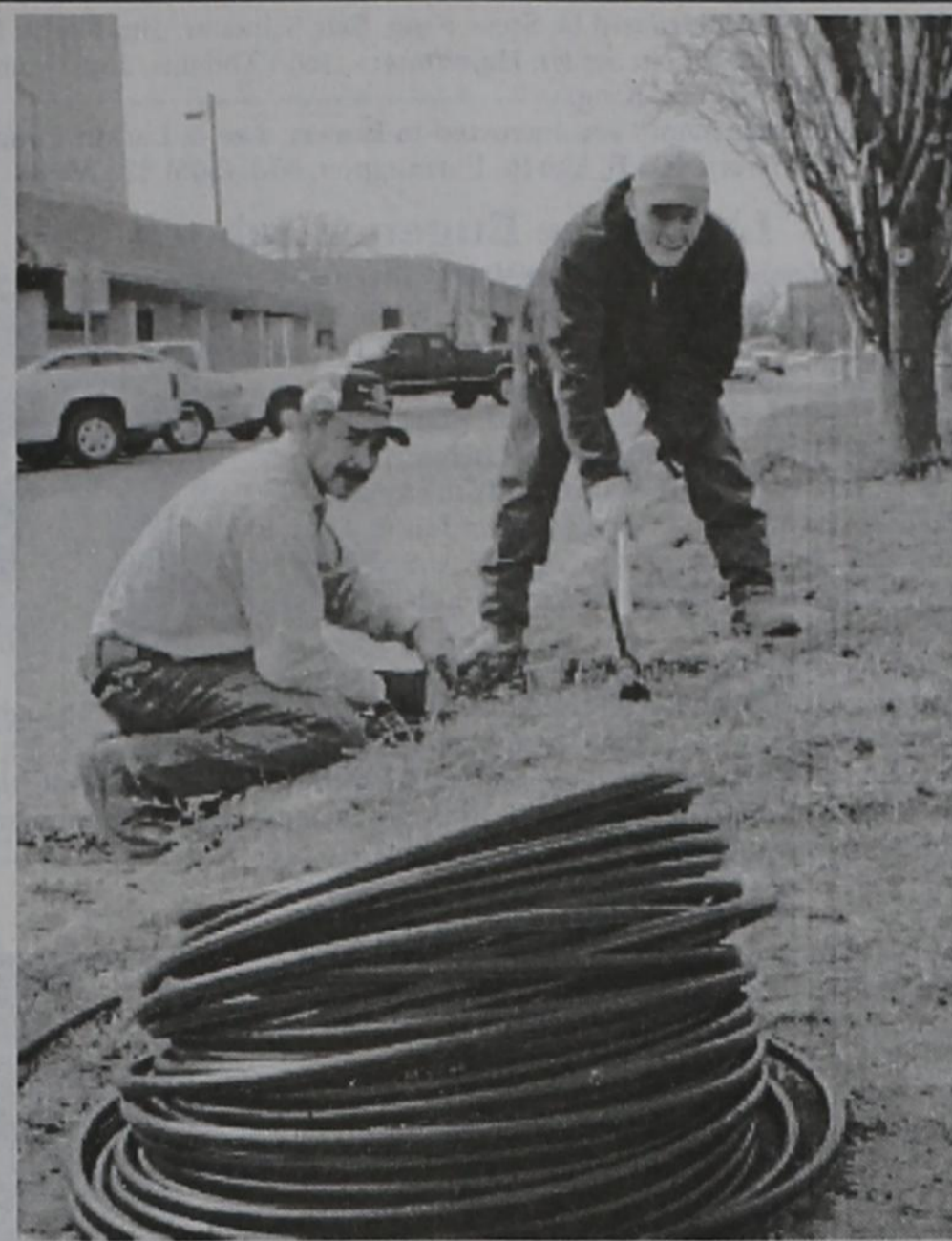
Frank Florez (left) and Brent Justice worked through the day with other city employees installing a new drip irrigation system on the East Main Street median. With hopes to avoid water waste, the crew was tasked on Monday not only to install new lines, but to cut out the old sprinkler system. (Staff Photo by Tim Burnett)
