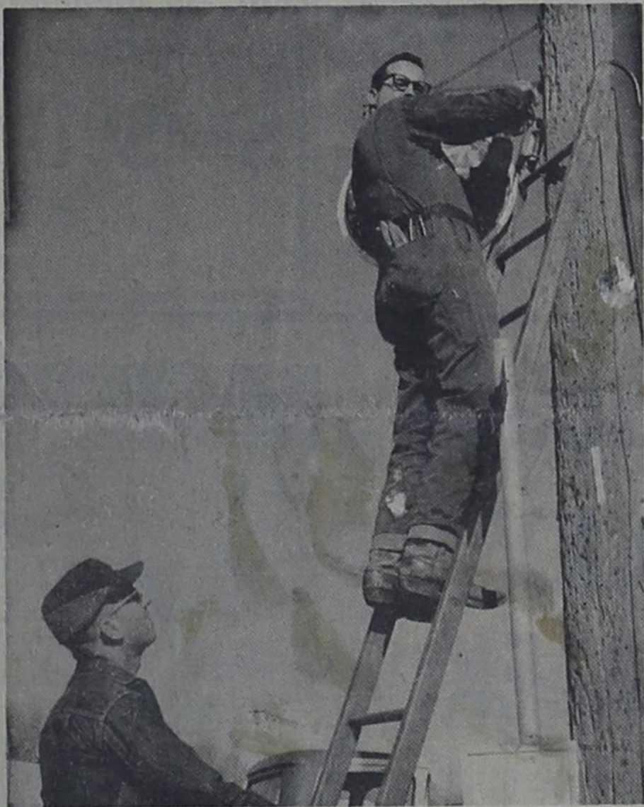
FIRST THE WORK -- Bovina Jaycees devoted many man-hours to the erection of Christmas lights and decorations in the downtown area. Alfred Moody is shown tying in an ornament to an electric line and Bob Fillpot steadies the ladder for him.
