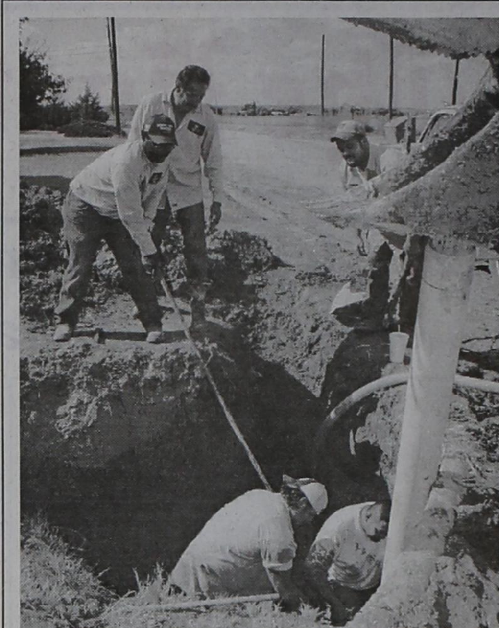
Repairing a six inch water main at the intersection of 15th and Sunset Dr. on Friday, October 14 are City of Post employees (ground level left to right), Owen Gilbert, Frank Flores and Lazaro Moreno (working in the hole left to right), Bryan Looney and Johnny Torres. According to Interim City Manager, Delbert Rudd, the 6" water line separated at the joints under W. 15th Street and the city crew had to pull the old pipe from a conduit and replace with new pipe. A long piece of pipe is shown being used to hold down the water line while the crew tightens the connections for the repair clamp. As a result of the repair job, water was cut off to approximately six homes on W. 15th Street through the day. (Staff photo by Tim Burnett)
