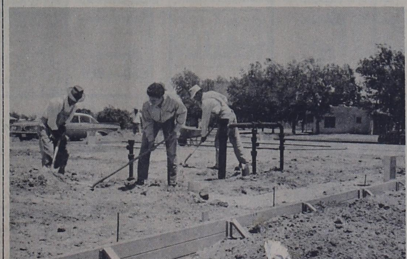
PARRISH HALL WORK --- Shown working on the foundation of St. Ann's new parrish hall which is now under construction are, left to right, S.A. Brito, Artemio Cano and George Cervantez. In the background is Antonio Gomez. The new hall is being built on St. Ann's property on Third Street.
