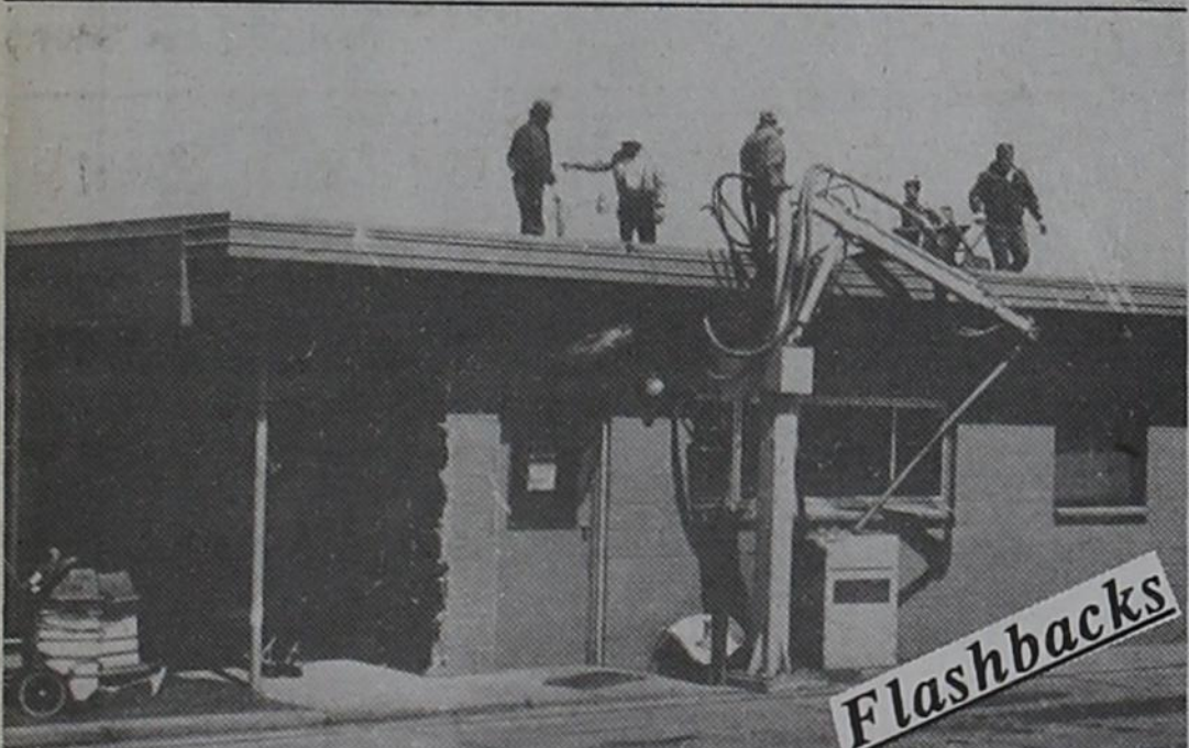
STORM DAMAGE --- One of the facilities hit by tornado-like winds last Friday night was the office building at Caprock Feeders. The building lost its roof, part of which is shown in the top photo. The bottom photo shows workmen on top of the building making necessary repairs.
