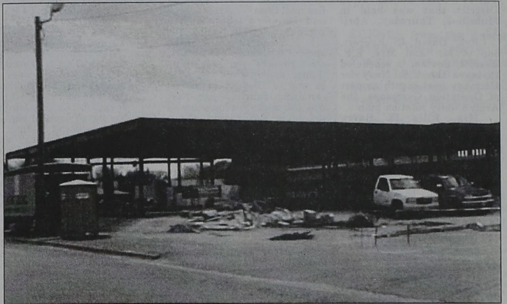
WORK CONTINUES on the expansion at Panhandle County Community Hospital in Friona. Workers raised the first steel at the site last weekend. ron carr photo
