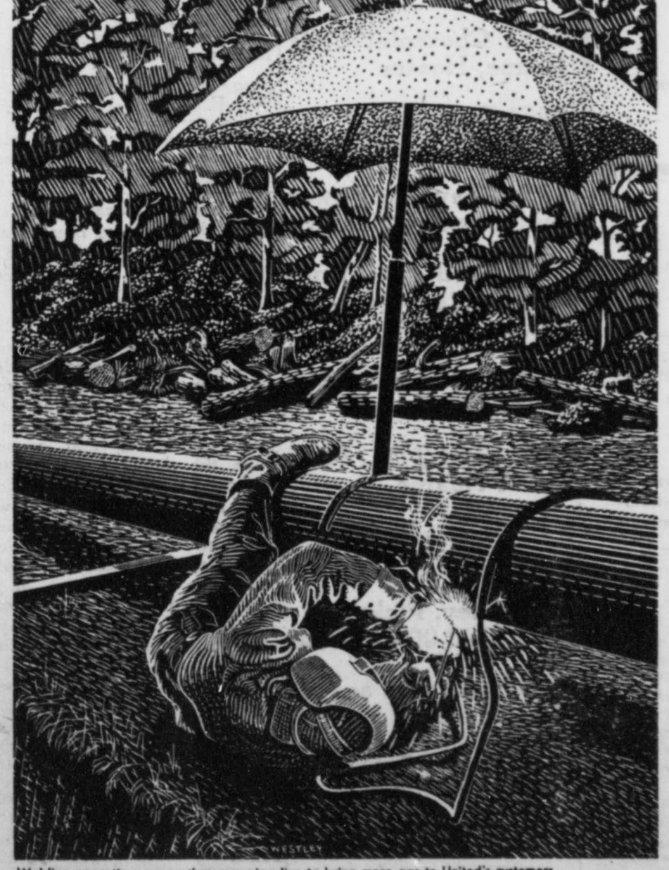
Welding operations on another new pipe line to bring more gas to United's customers
