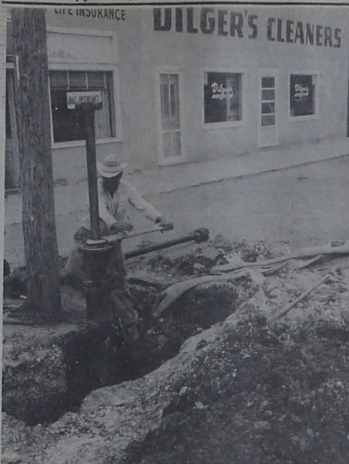
WATER TROUBLE -- Andy Garza, city employee, and Water Superintendent Paul Holcomb, not shown, repaired a leaking fire hydrant at the intersection of Third and Main Streets Friday. The repair work caused water to be off in the downtown area for a period of time Friday afternoon.
