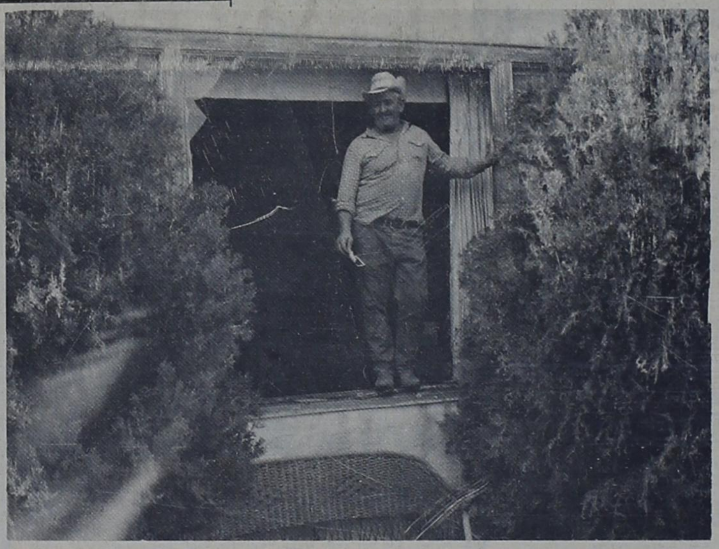
WIND DAMAGE -- Cecil Sisk stands in what formerly was the picture window in his home. Other damage was also done to the home by high winds last week.
