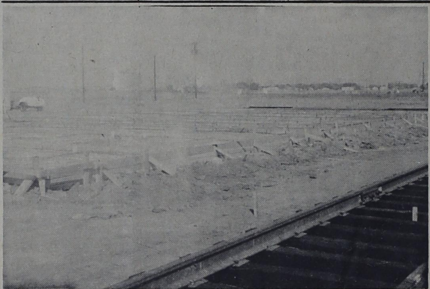
NEW BUSINESS -- Forms for the foundation for the new building for Cynanamid farm supply center were in place the first of the week. The structure will be 50 by 120 feet in size. A portion of the town may be seen in the background.
