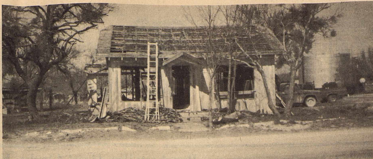
This old building, located across the street from the B.I.S.D. School, is being torn to the ground. The building and lot are property of Happy Shahan.
