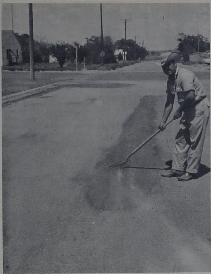
PAVING PATCHED -- Andy Garza, a member of the staff of the City of Bovina, displays a recent patching job which was done on a paved street here. Holes in the streets are being filled in preparation for seal coating of some 40 blocks of paving. The seal coating work is scheduled to get underway next week. City workmen have been doing the patching.
