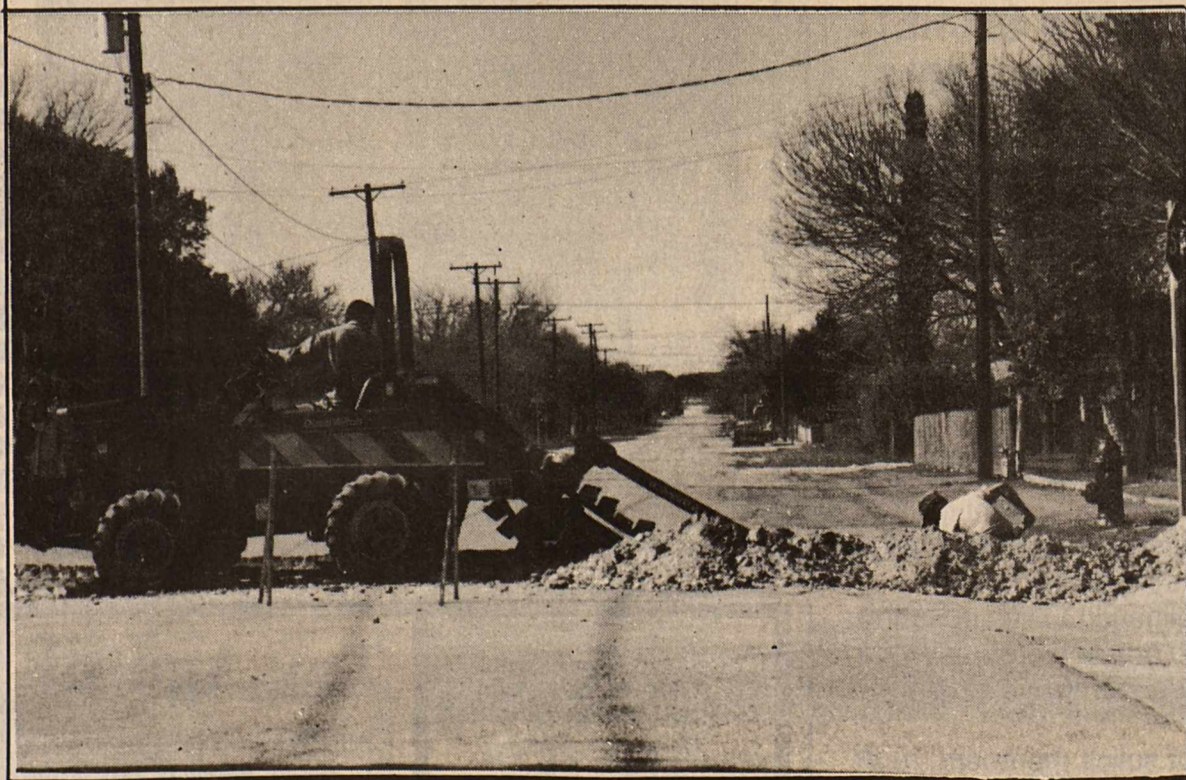
The telephone system in Brackettville is being upgraded. The work is being done by Dynatren Construction Company of Uvalde. Ruben Colunga trenches while Ronnie Calloway helps. Fort and 3rd Streets.
