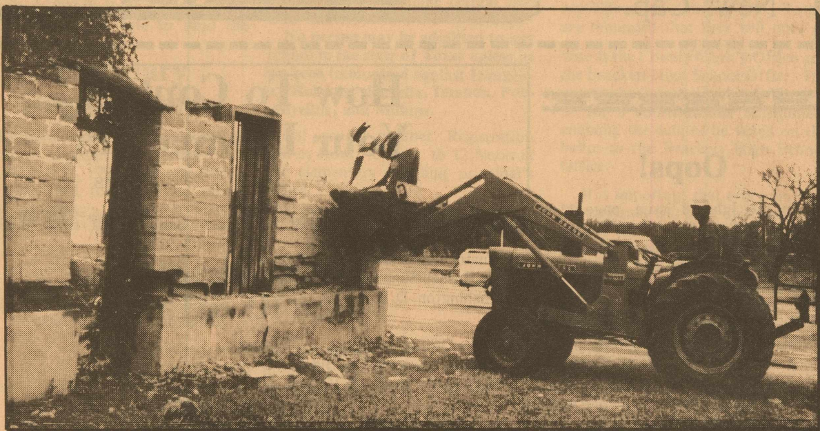
Baltazar Espinosa and his assistant, Manuel Licea, dismantled the wall fragments of the Mellifont Building. They have now completed the task by numbering and storing each rock which will be used in the Library Expansion Project.
