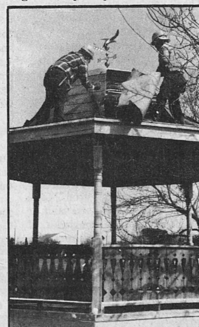
Bandstand - The bandstand at Fort Clark received a copper roof this past week-end virtually completing the project. Reggie Acosta and another employee (unidentified) of Beldon Roofing Company, San Antonio, are shown working on the project.
