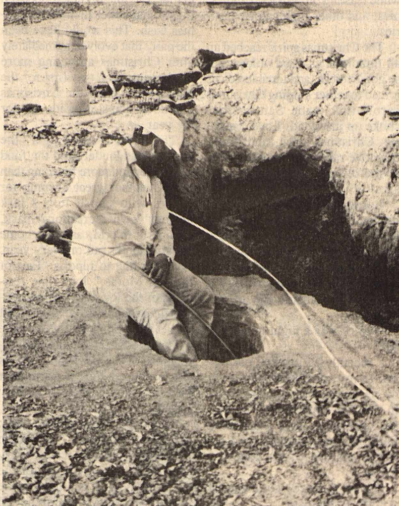
George Corral, who works with Holloman Construction out of Odessa, works on the city's new sewer system Wednesday on Ann Street.
