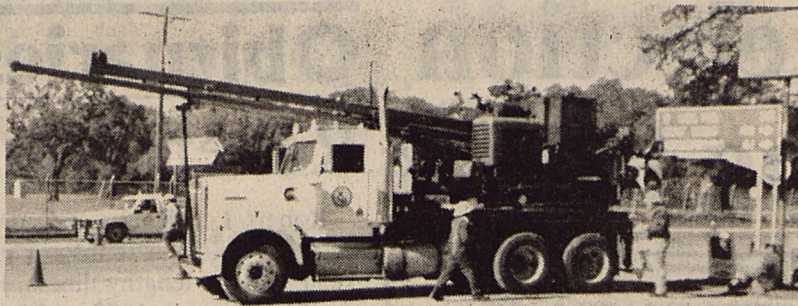
Texas Department of Transportation crews have begun installing the new stop light at the intersection of Highway 90 and Ann Street. Brackett News Photo by Jewel Robinson
